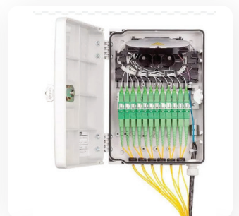
Wall Mount Patch Panel
